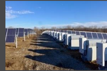
FAIRFIELD/IOWA 1 MWh, 32 VFBs
